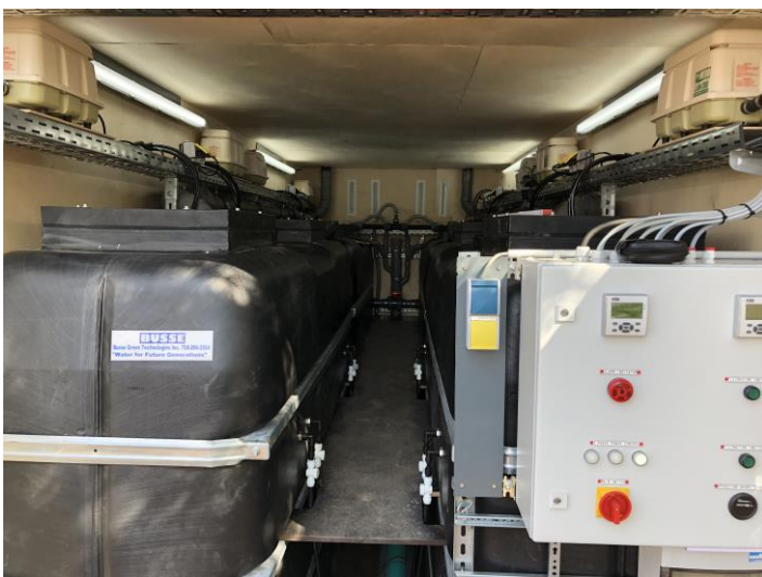
View into the interior of the container. A footbridge between the rows of tanks enables trouble-free work at the blowers fixed above the tanks. It also guarantees access to the membrane modules, which are installed in the tanks.
