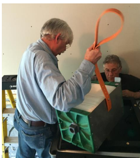
Membrane disc module being installed in the BUSSE-system by Mr. Schaefer (BUSSE Green Technologies Inc) and Mr. Fred Lambiase (Busse New York Inc.)
