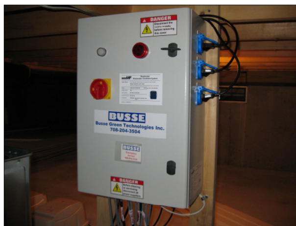
Control unit of the system
