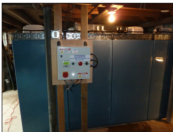
Control unit of the system
