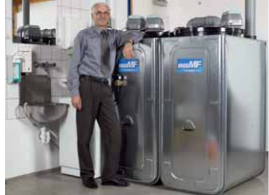
Plant type GT 220, installed in a cellar
