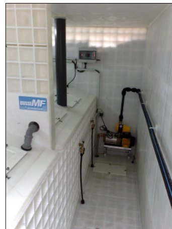
Waste water treatment system, feeding pump
