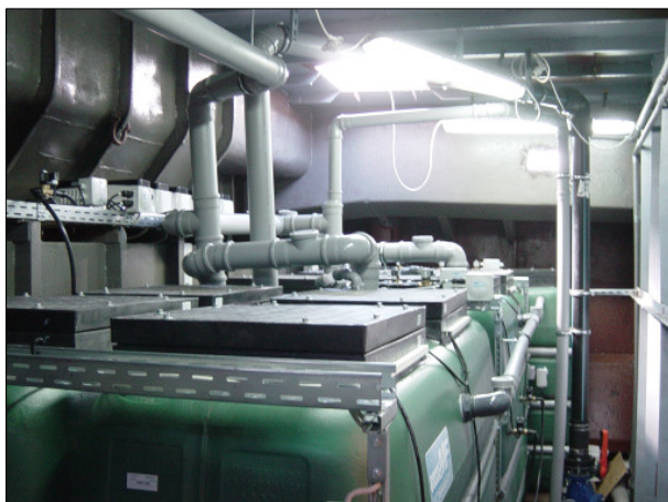
Waste water treatment system
