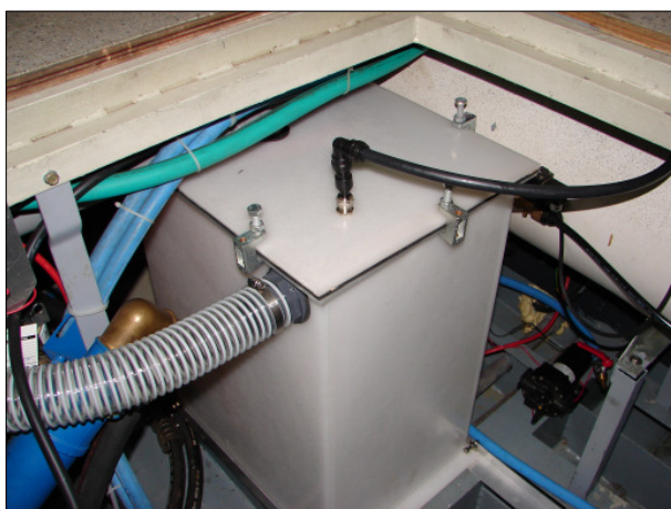
Membrane biology reactor in the engine room
