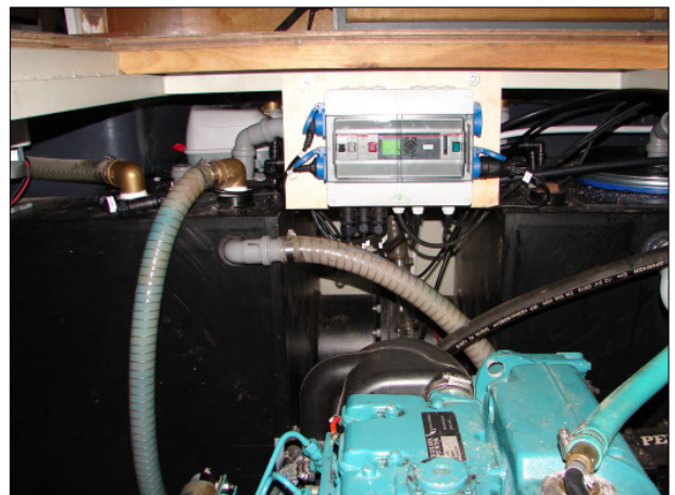
Sewage and aeration tank with control unit
